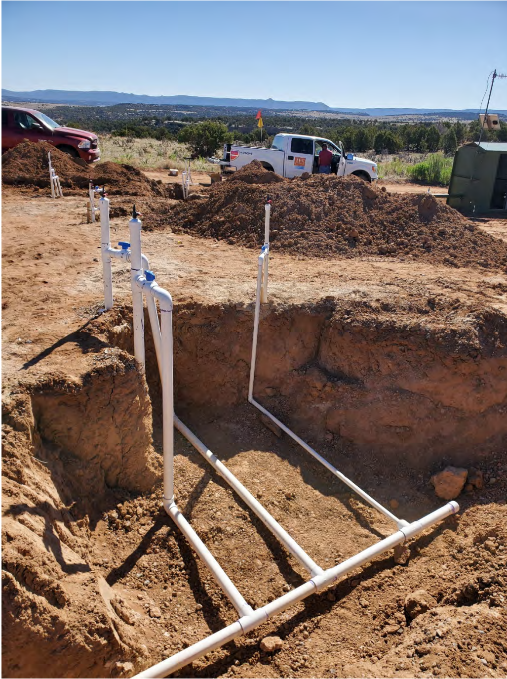
Photo 4: SVE piping connection setup to SVE wells.
