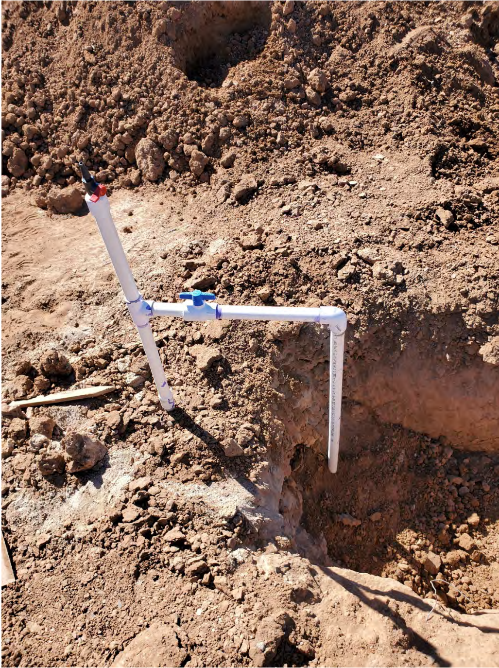
Photo 3: SVE piping connection setup to SVE wells.
